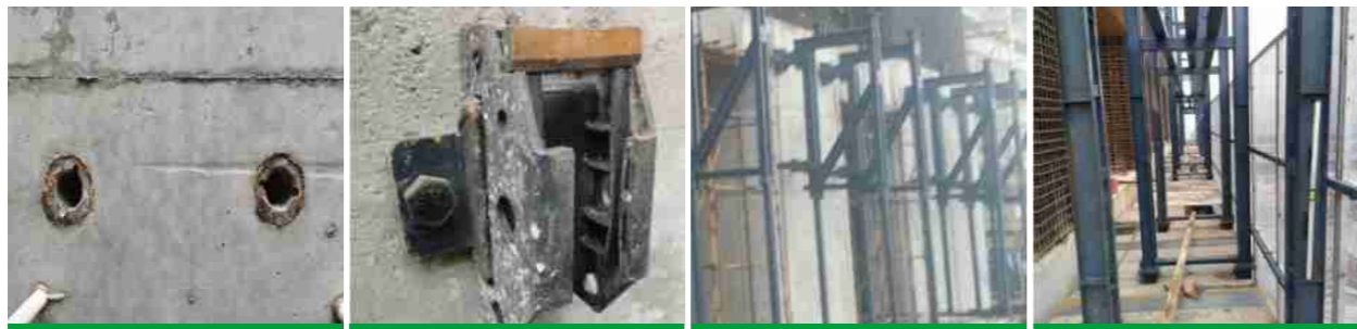
■ 放置爬模埋件 Place the Buried parts ■ 安装附墙装置 Installation of Attached Device ■ 安装爬模架体 Installation of the Frame System ■ 安装爬模平台 Installation of the Platform
