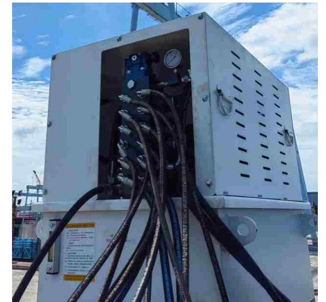
泵站 Pump station
